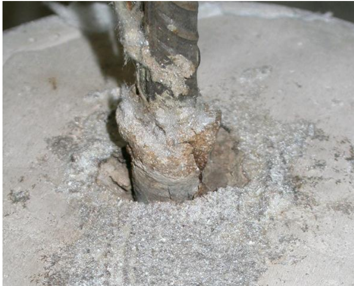
Figure 8: Bond failure after fire exposure
